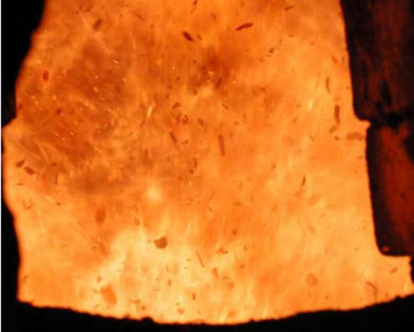
Too Much Underfire, No Overfire, High CO, Poor Combustion
